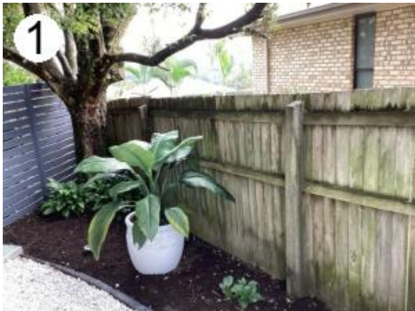
#1. Various wood decay and deterioration / movement has occurred to the timber fencing around the perimeter of the property. A further detailed investigation by a competent person, e.g. a licensed building / fencing contractor is recommended to determine the cause, method and extent of any remedial work required, and associated costs. The above recommendation should be implemented as soon as possible.
