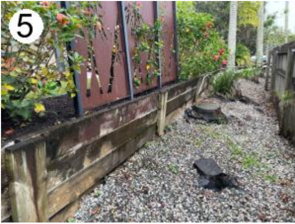
#5. Various wood decay and deterioration / movement has occurred to retaining wall timbers. A further detailed investigation by a competent person, e.g. a licensed building contractor / retaining wall specialist is recommended to determine the cause, method and extent of any remedial work required, and associated costs. The above recommendation should be implemented as soon as possible.
